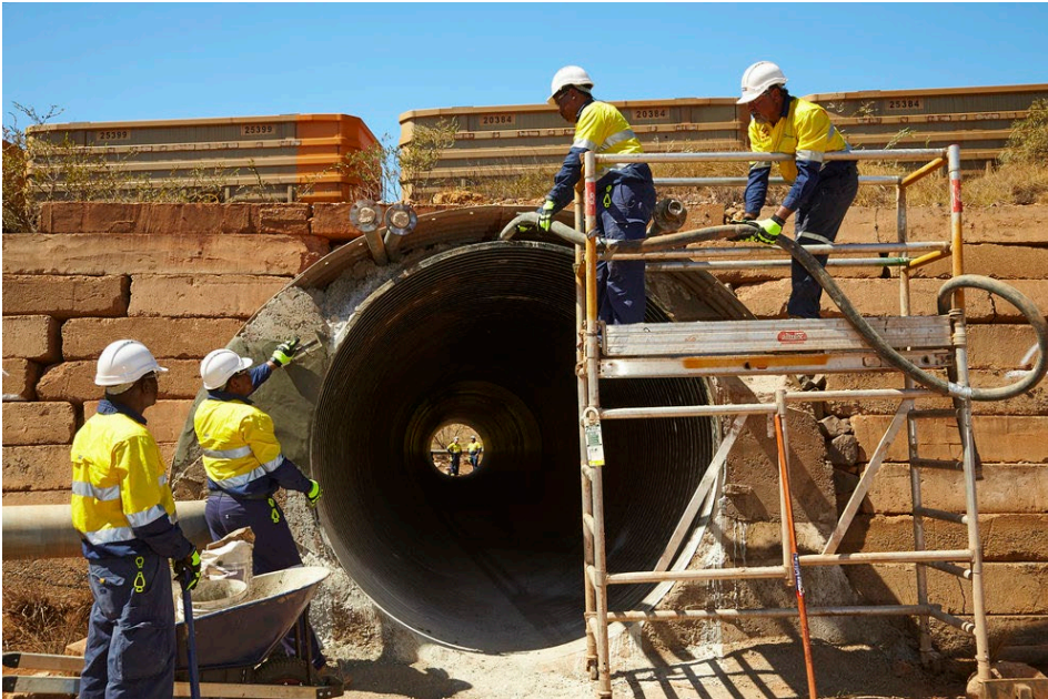
Figure 5 Yurra's Rio Tinto Iron Ore railway culverts relining contract Photo courtesy of Yurra Pty Ltd
